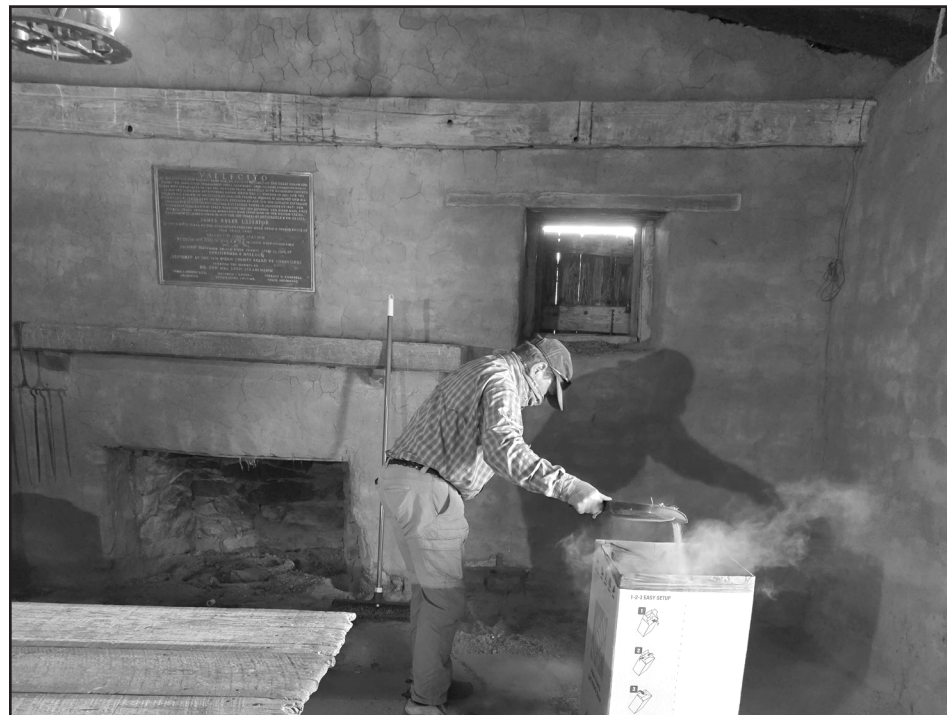
After cleaning out years of dirt and other debris, the stage station is ready for more restoration work.
